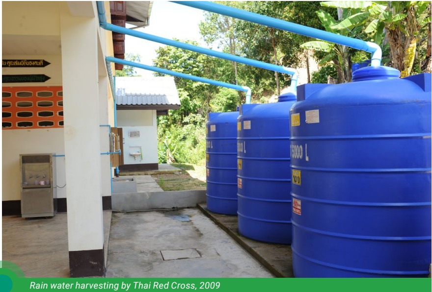
Rain water harvesting by Thai Red Cross, 2009
